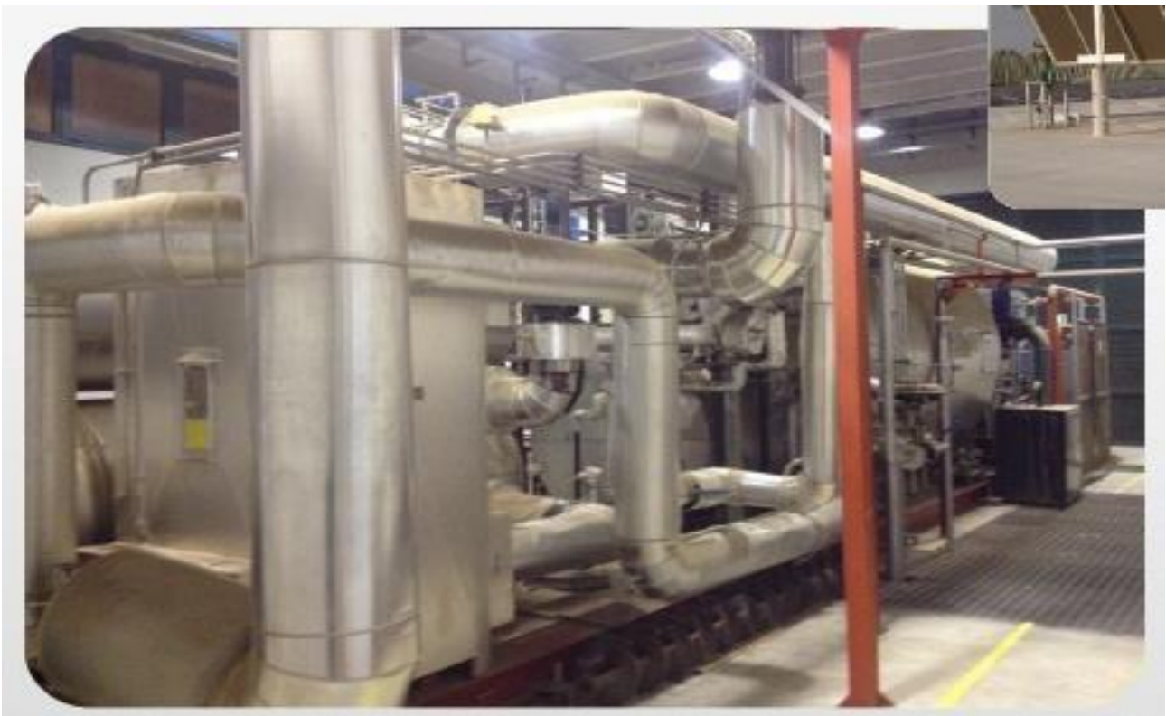
Figure 7 - The 1MW ORC turbine
