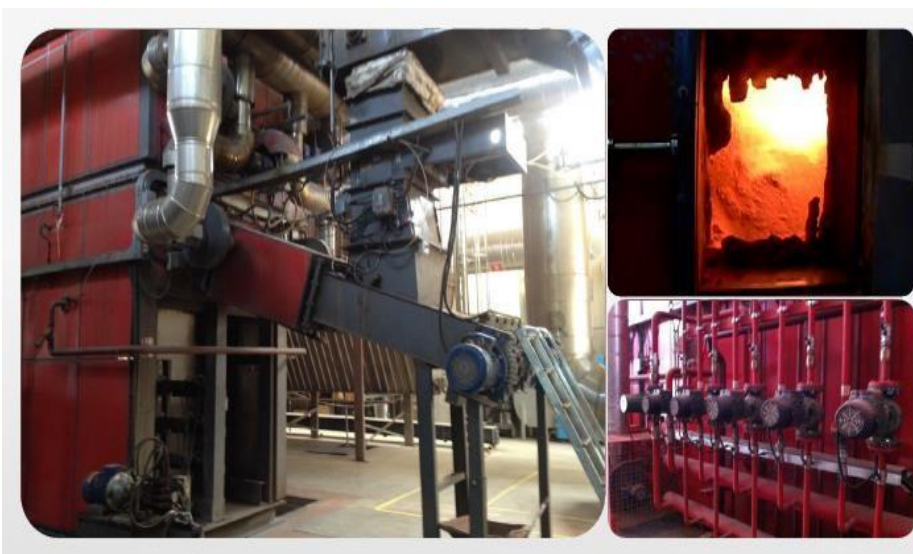
Figure 6 - The 4.4 MWth moving grate boiler
