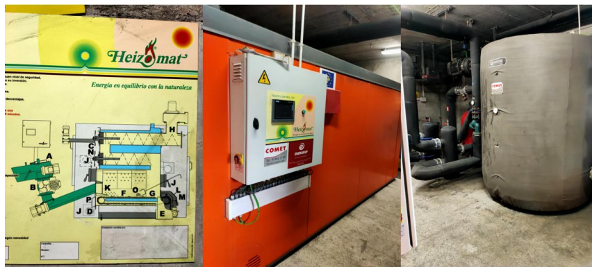
Figure 10. Boiler and district heating system.
