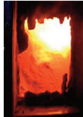
FIGURE 6. The 4.4 MWth moving grate boiler
