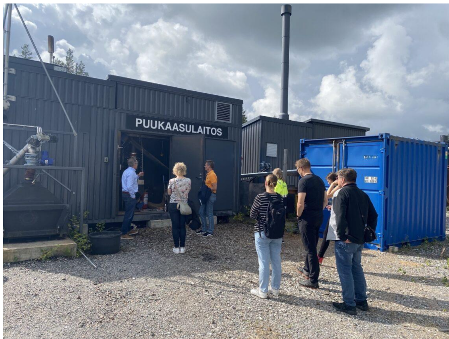
Picture: Wood gasification experimental facility. The process gained a lot of interest among the participants and contact information were exchanged for potential cooperation in the future related to oxygen-enhanced gasification process.
