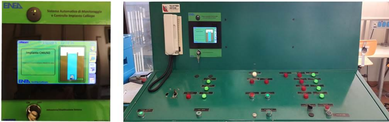
Figure 8 - a) Touch screen display and b) monitoring and diagnostic automatic system installed on the Calliope facility control console in the control room.
