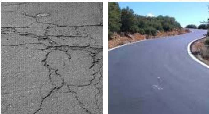
Cracked Conventional Asphalt and Rubberised Asphalt after 3 years of use Nea Makri (Athens)
