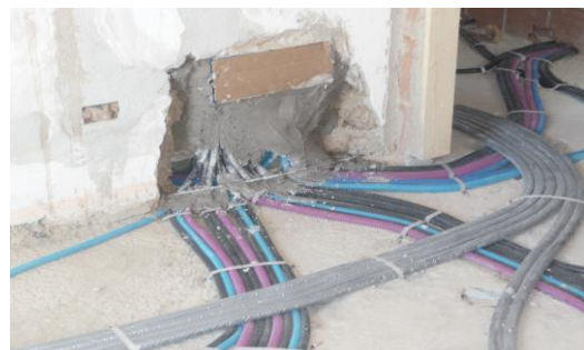
2014 - Electrical Equipment supermarket
