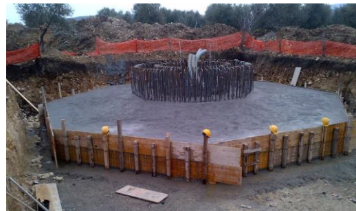
2014 - Wind Power Plant Deliceto (FG)
