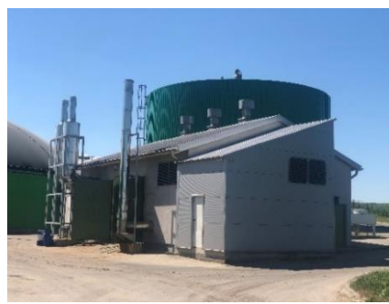
Figure 2. Cogeneration block at Biogal. Source: BIOGAL
